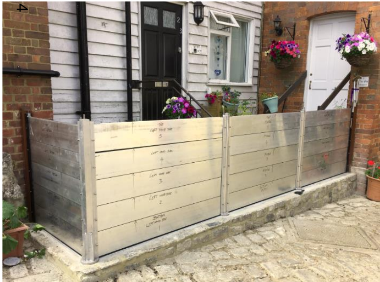
Flood barriers reducing risk to 3 properties
